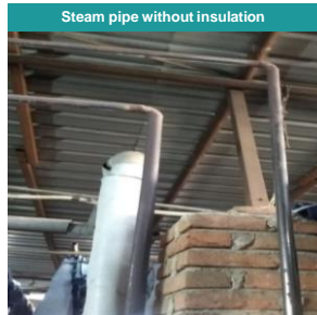
Steam pipe without insulation
