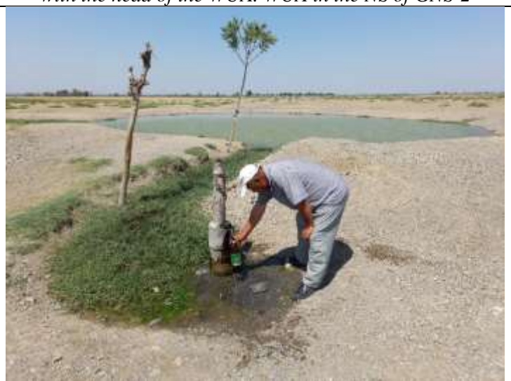
Drilled well in the Zafarabad district
