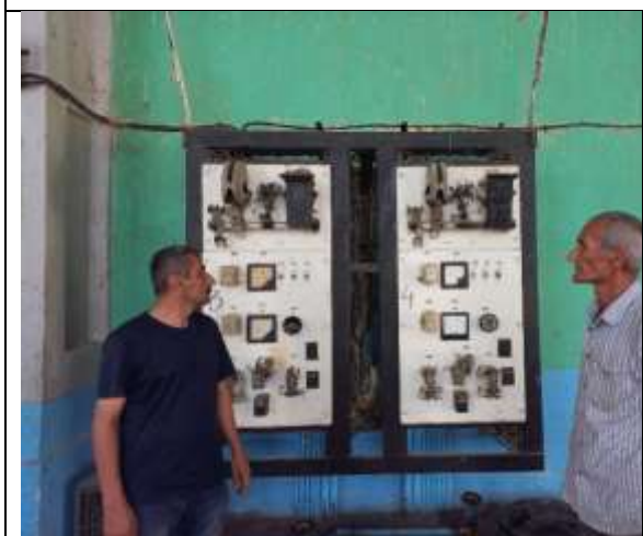
Meter inspection at HNS-2
